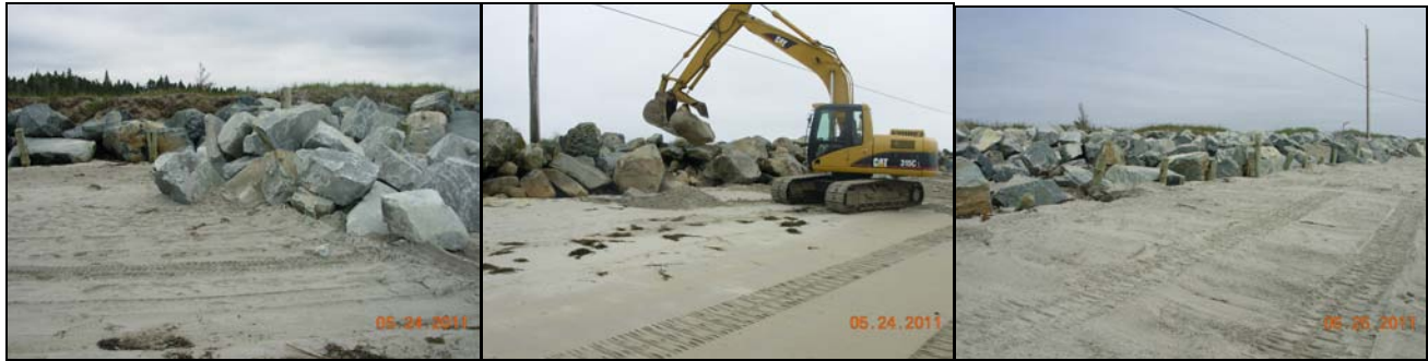
Left: The first load of rock is delivered (note the exposure of the dunes in the rear). Middle: Rocks being individually placed into the cribwork. Right: The finished product! All photos courtesy of Mary Fulleman
